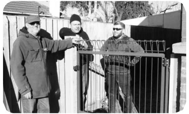
North Dunedin Shed Society members installing a new gate at the Dunedin City Toy Library.
