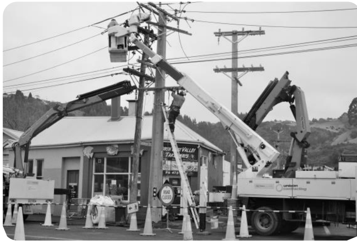
Workers installing new power poles near Northeast Valley Normal School as part of Aurora Energy's Fast Track pole programme.
