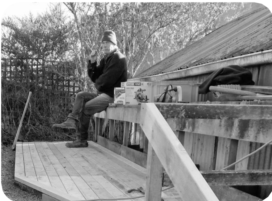
North Dunedin Shed Society's hard working president Wayne Jefcoate taking a well-earned break after a deck rebuild and before concreting the steps.
