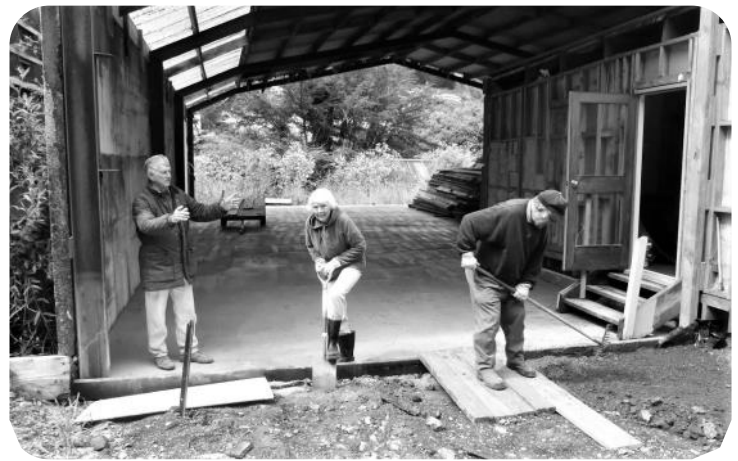
From left, Norman Ashbury, Kirsten Ashbury and Jim Gladding working hard at 'The Shed' before the installation of the end doors.
