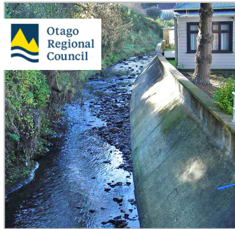
A section of the Lindsay Creek channel in North East Valley (looking upstream). Note the narrowness of the channel, the steepness of the true right (vegetated) bank and the proximity of the houses and yards. (The concrete channel lining and floodwall are ORC assets.)
